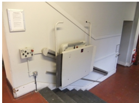
First Floor stair lift
